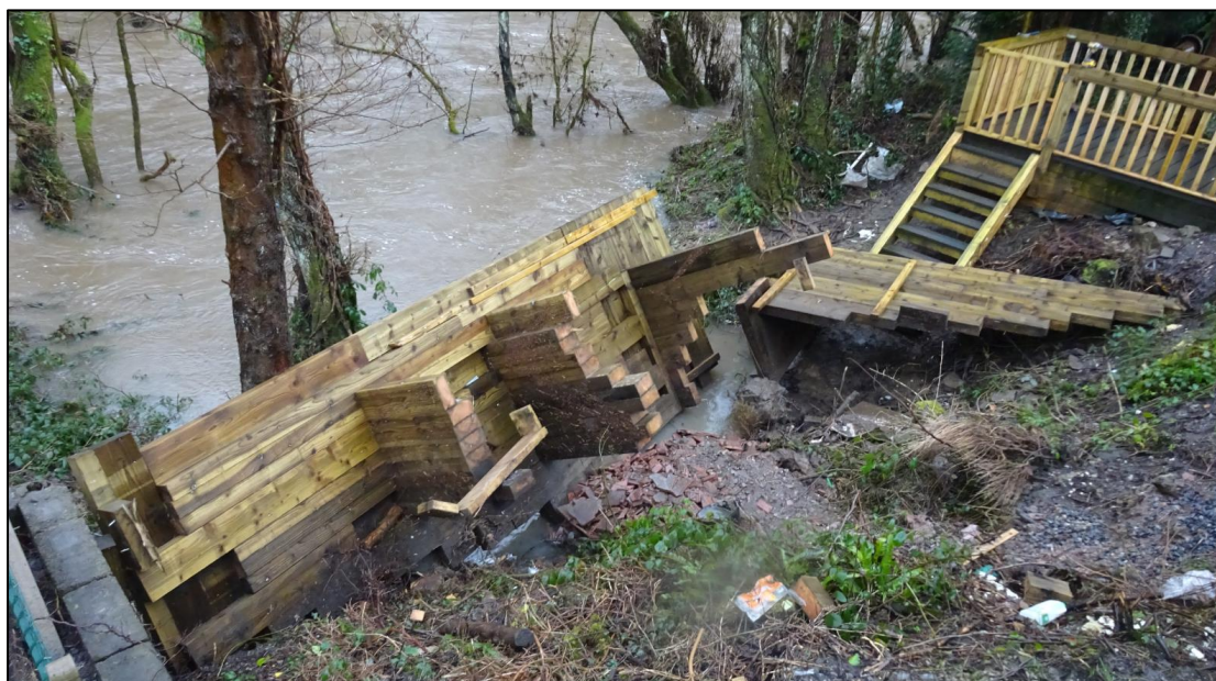
Figure 14: Damage to property caused by the River Cynon to the rear of Richmond Drive, Hirwaun on the 16 th February 2020 (image captured by resident)
