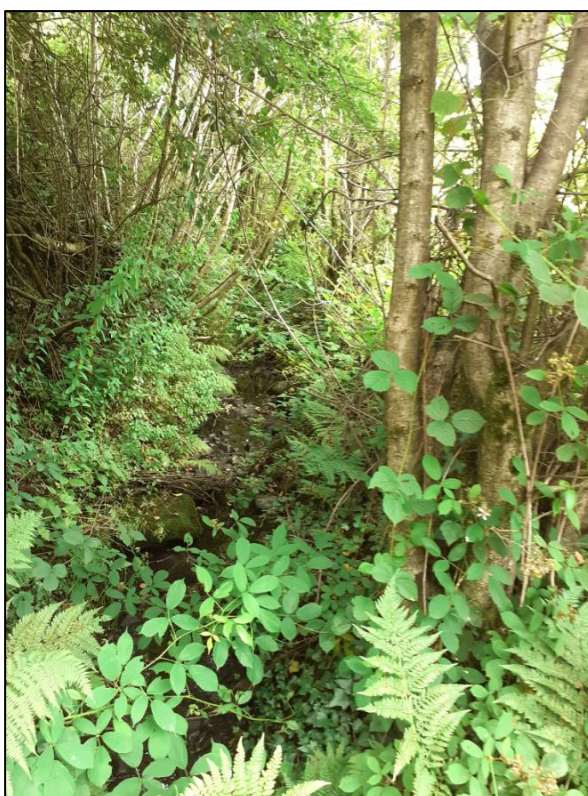
Figure 11: Undefined and overgrown ordinary watercourse channel above Meadow Lane Culvert Inlet 2 (image captured by RCT's Flood Risk Management team following Storm Dennis)
